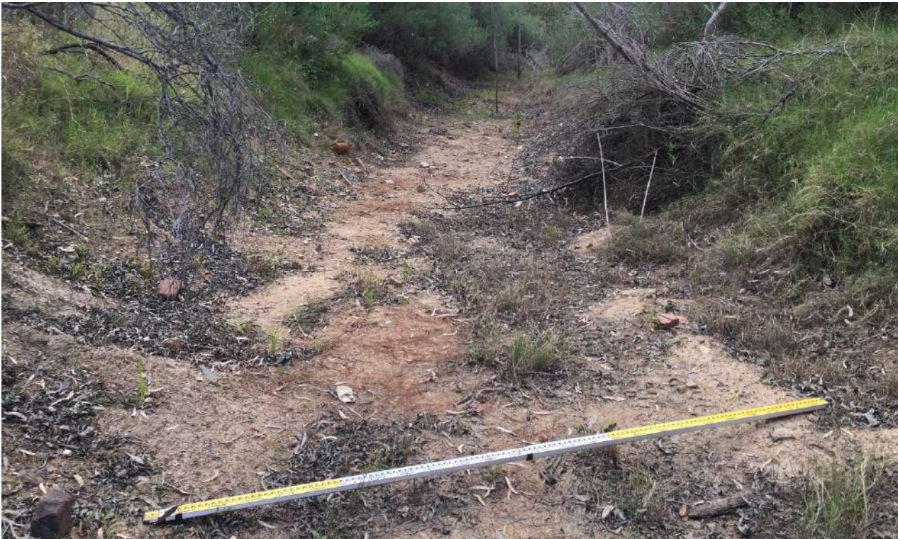
PLATE 20: Open drain to southern outlet (In process of decommissioning as part of Area 3 Stage 5 works)
