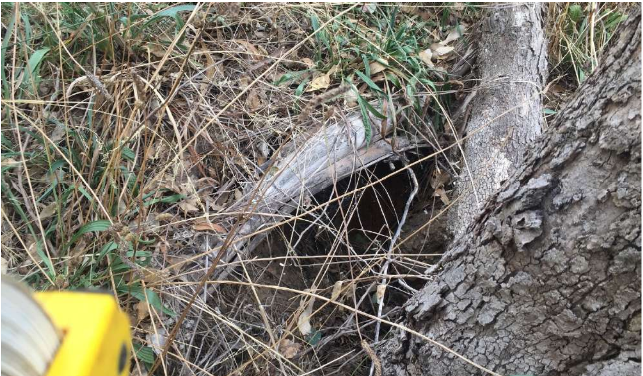
PLATE 6: 400mm dia steel culvert under driveway largely blocked by large tree and sediment.
