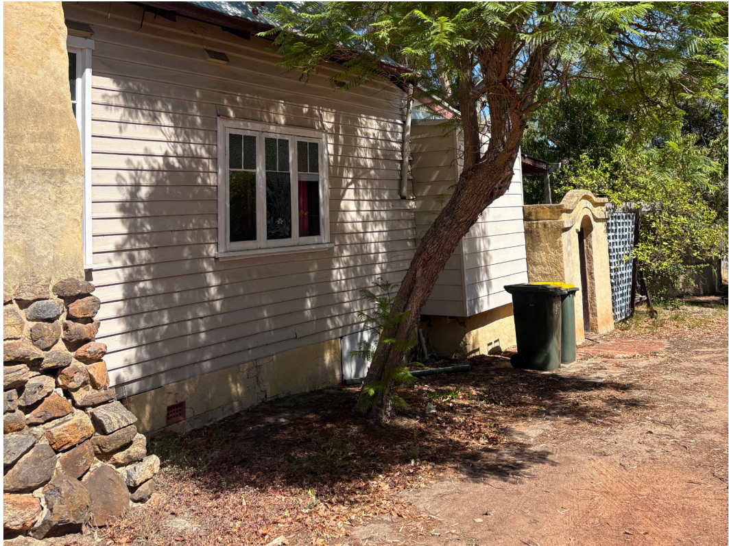
Figure 19. Side (north-east) elevation of residence, showing proximity of Jacaranda tree, causing damage to residence. Damaged weatherboard cladding proposed for replacement. Note disconnected downpipe (DAR Studio, February 2026).
