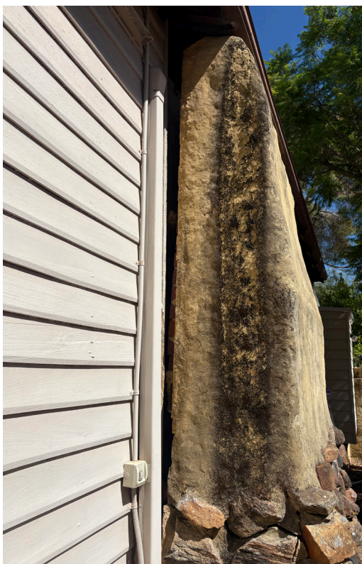
Figure 13. Detail of chimney detached from the house (DAR Studio, February 2026).
