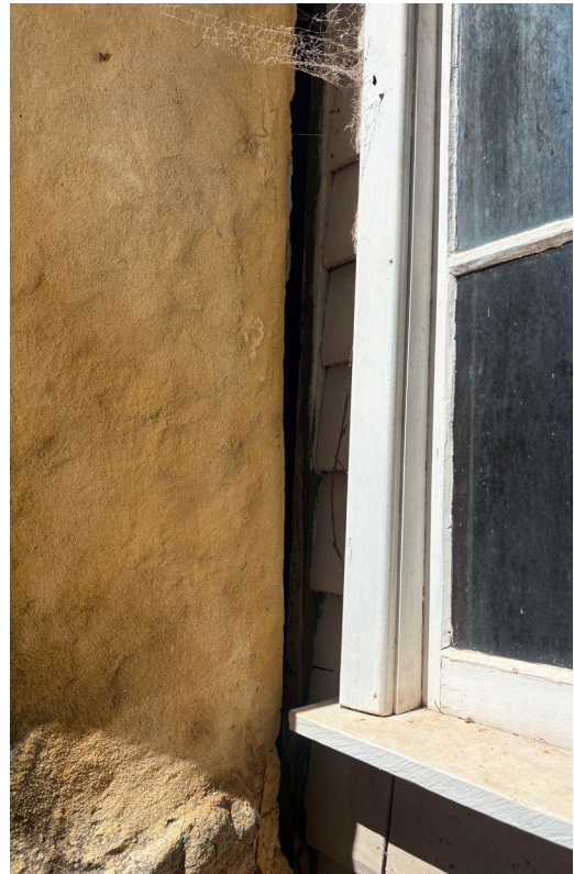
Figure 14. Detail of chimney detached from the house (DAR Studio, February 2026).
