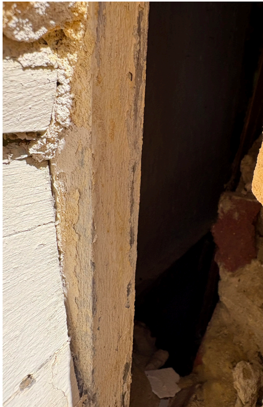
Figure 15. Significant detachment of chimney (DAR Studio, February 2026).
