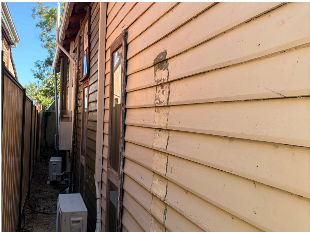
Figure 20. Side (south-west) elevation showing mis-matched and damaged cladding proposed for repair and replacement (DAR Studio, February 2026).
