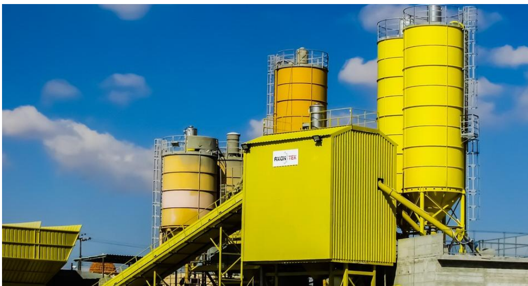
Figure 7 A typical concrete production facility, which comprises several energy-intensive processes.
