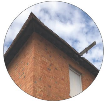
Original openings to the north elevation will be reinstated. Upgrades to the roof including guttering and downpipes consistent with the original architectural style will be adopted to mitigate issues such as rising damp.
